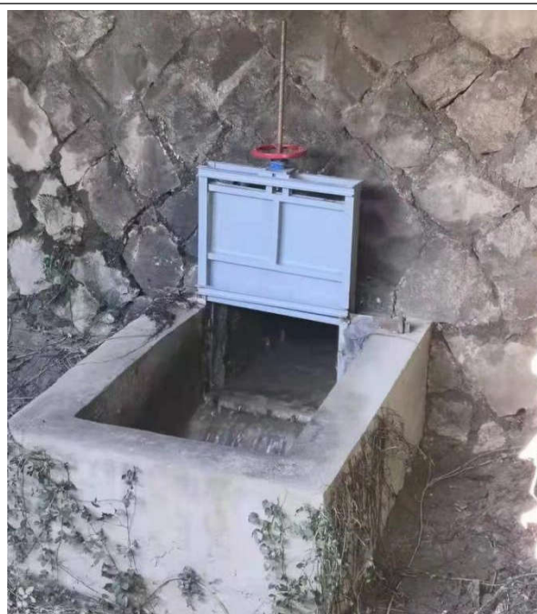
污水处理二站雨水口水闸
